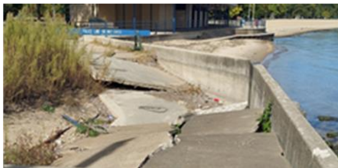
Shoreline damage at Calumet Park (above) will undergo reconstruction in 2026.
