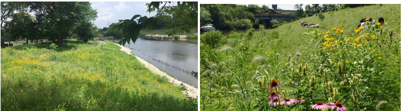
Riverbank restoration underway at River Park (left) and completed at Horner Park (right).
